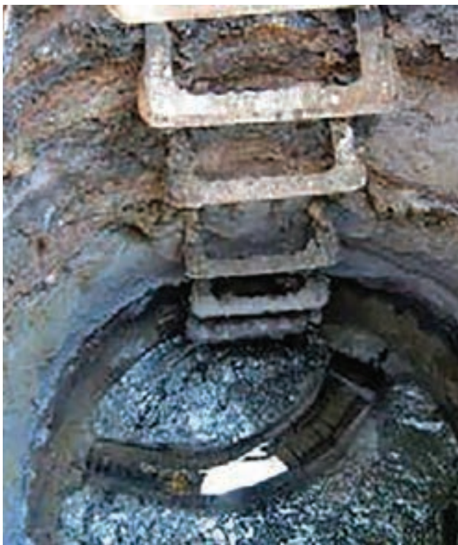
Figure 1: Corroded iron steps in a conventional maintenance hole.
