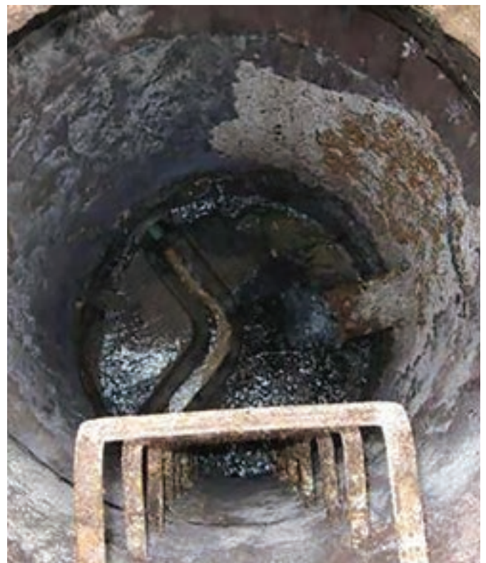
Figure 2: Sulphuric acid corrosion in a conventional maintenance hole.
